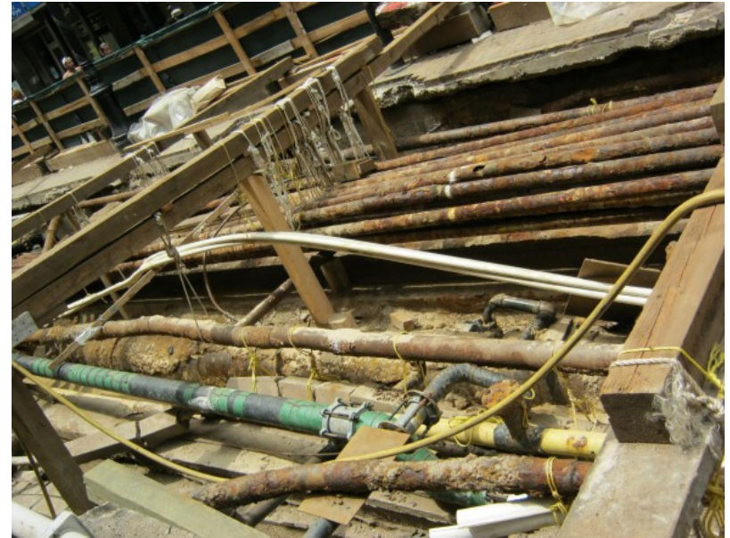
Underground utilities in NYC - www.balkanplumbing.com
