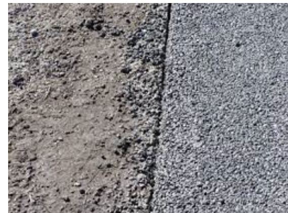
Clogged porous pavement - Charter Enterprises Inc.
