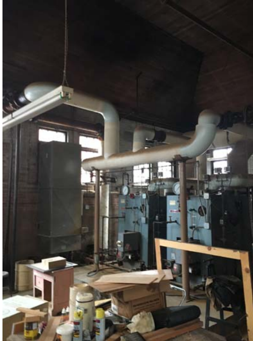
Figure 3-3. Inside view of power plant (as of Spring 2017).
